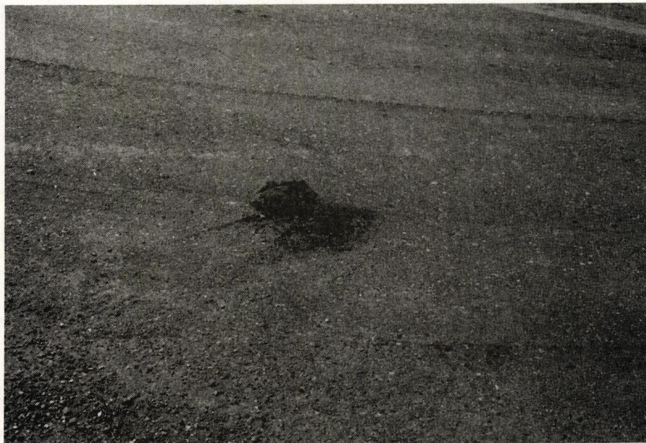
The truck seen backing into the side road in the top photo caused the damage shown below by turning his steering axle while stationary.
