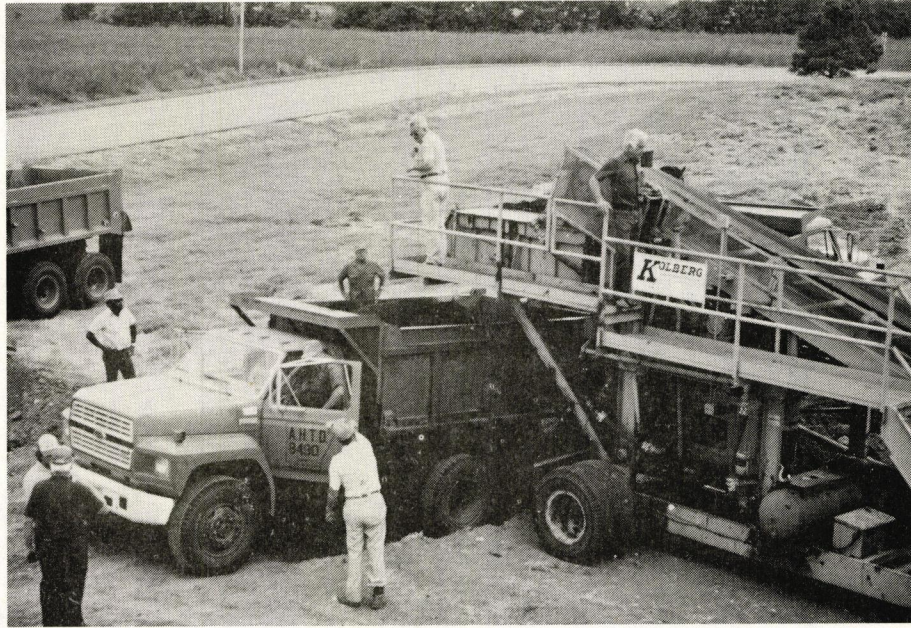
Field adjustments were made in the amount of water and emulsion added as necessary due to stockpile variability.
